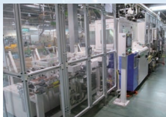
Automatic process line
